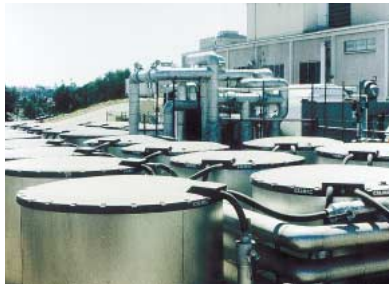
Owner: Grossmont Hospital, La Mesa, CA. Engineer: Verle A. Williams & Associates San Diego, CA. Contractor: Astro Mechanical, San Diego, CA.
