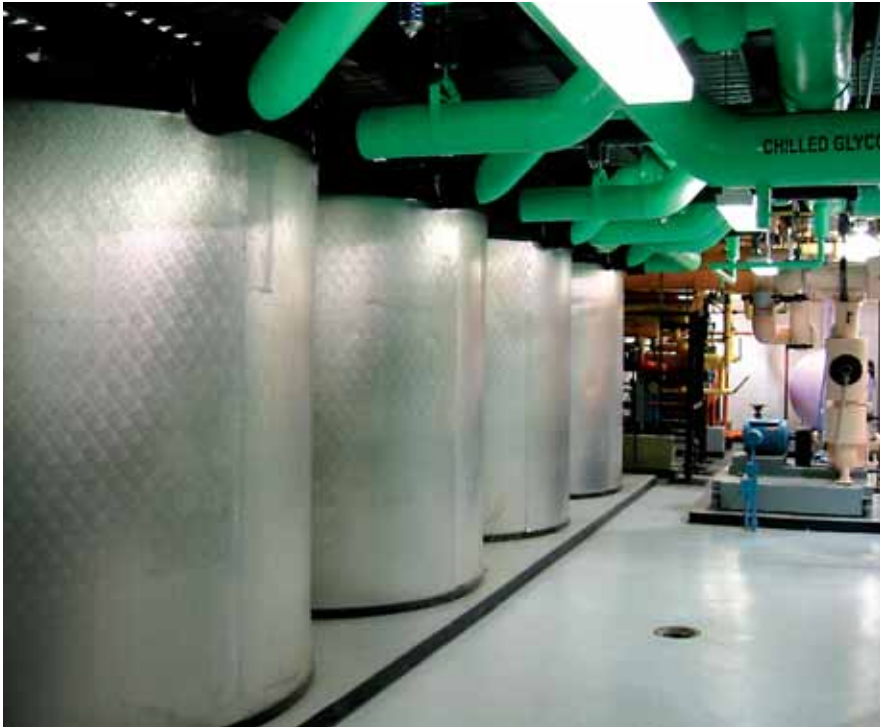
Many financial organizations in New York are turning to ice storage systems that use stored ice to augment the next day's cooling demand during peak periods.
