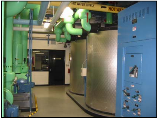
20 of the 28 tanks were put in the existing mechanical room, thereby using very limited rentable space.
