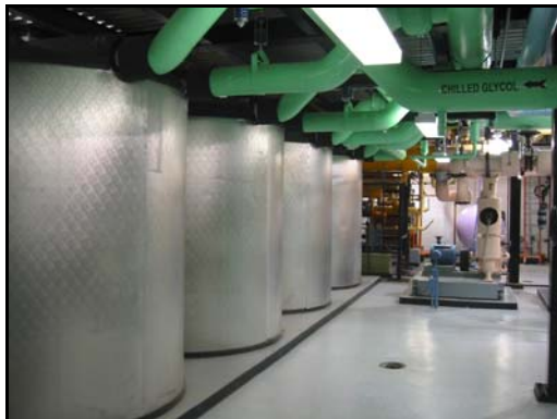
IceBank® Off-Peak Cooling tanks located in basement
