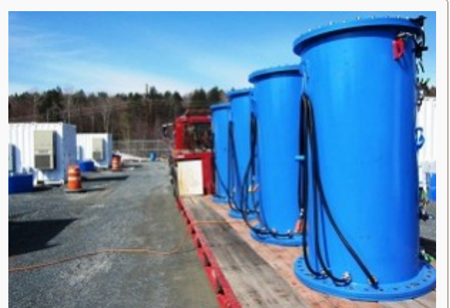
Some of Beacon Power's flywheels.
