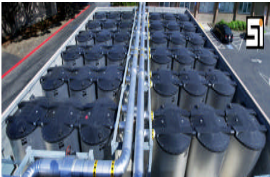
EQUIPMENT: TWO 600 TON HIGH EFFICIENCY CENTRAVAC CHILLERS WITH VFD AND 36 CALMAC ICE TANKS
